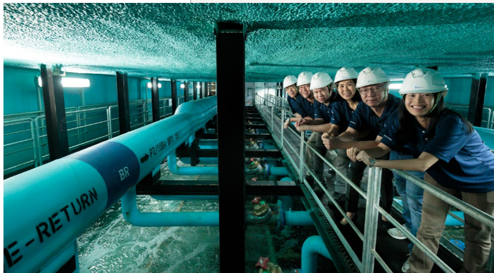
With two district cooling plants at Marina Bay Sands and One Raffles Quay, chilled water is centrally produced to support air-conditioning systems in buildings in the Marina Bay area, helping them save energy and cost.
