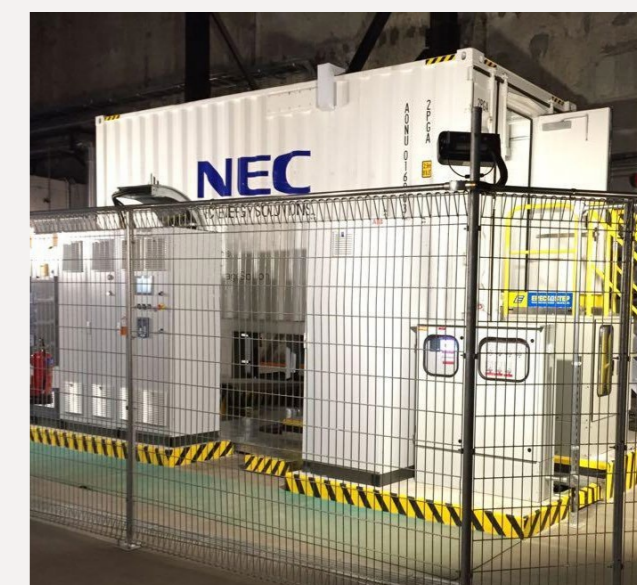
Underground ESS deployment for district cooling at Marina Bay area
