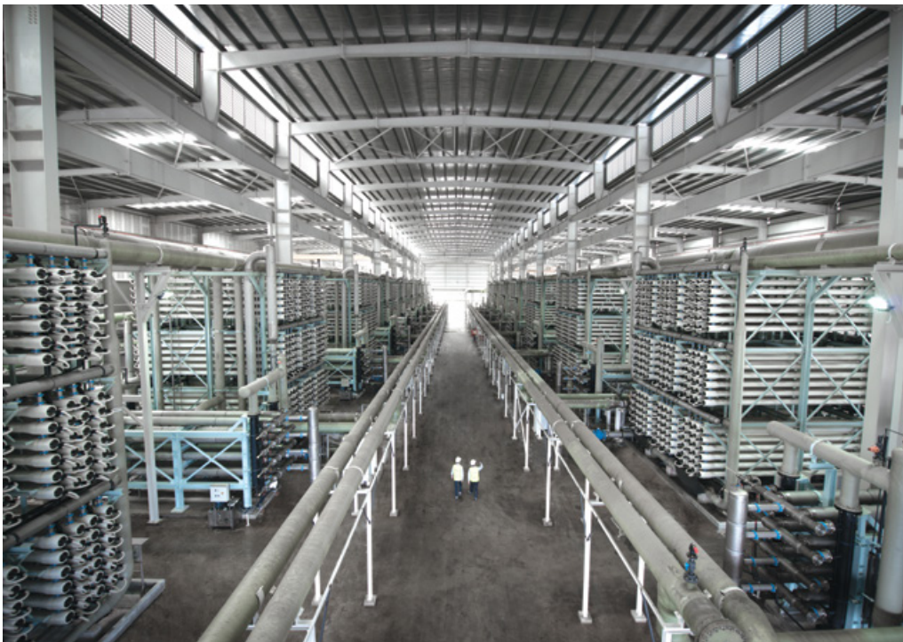
Tuaspring Desalination Plant
