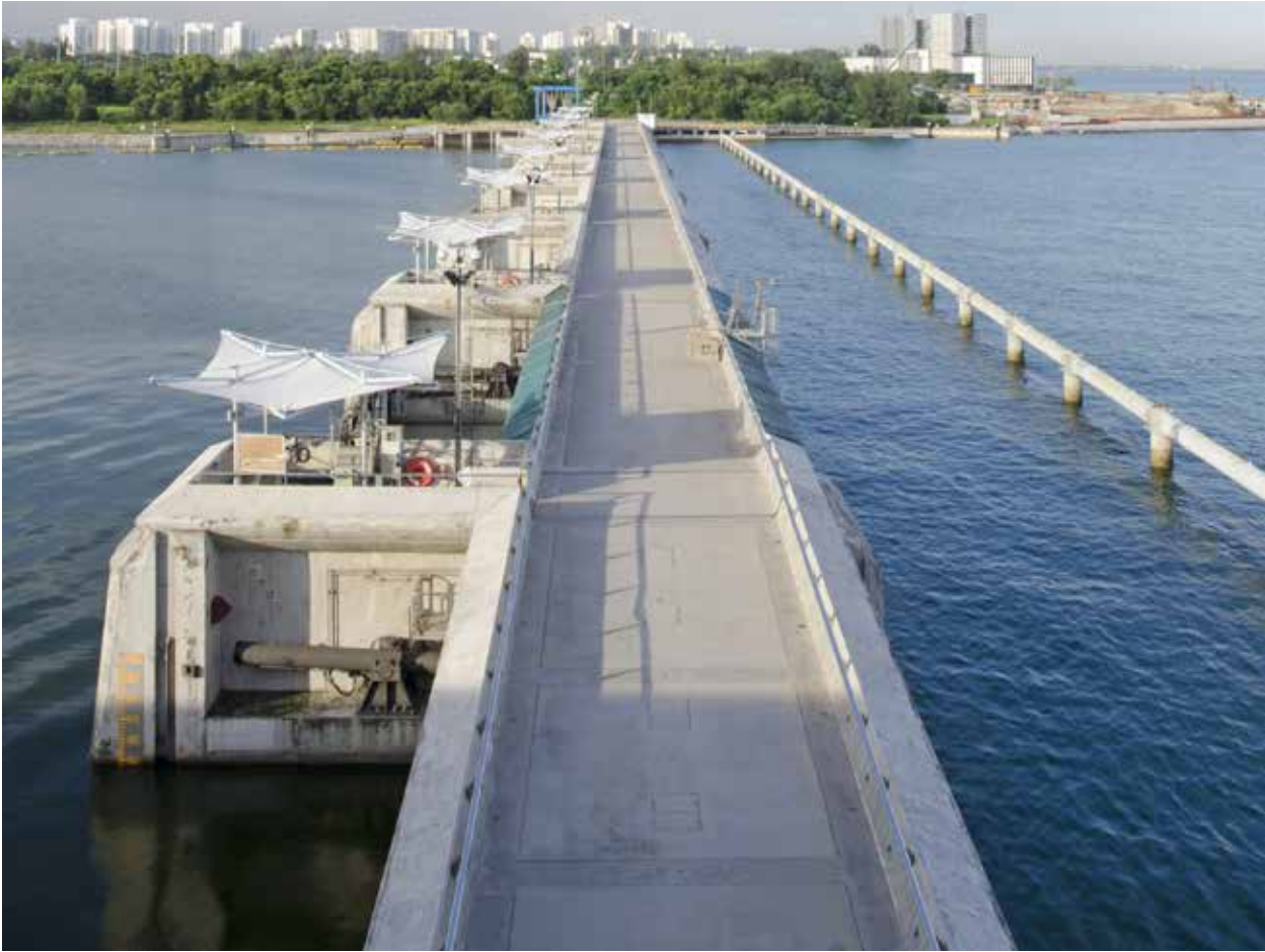
Crest gates at Marina Barrage are lowered when it rains heavily during low-tide to release excess water from the Marina Reservoir into the sea.
