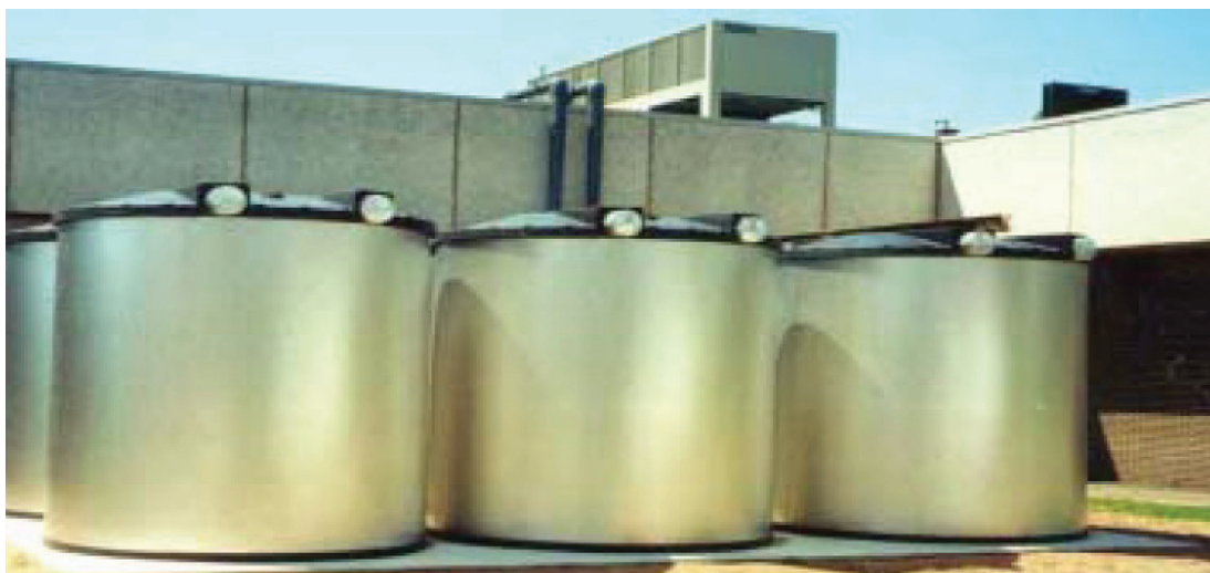
Figure A14: Thermal Energy Storage System Tanks
